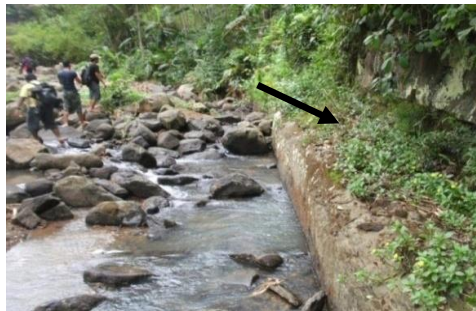
Fig.4. The appearance of a fault (Source: Suwarno, 2014).
