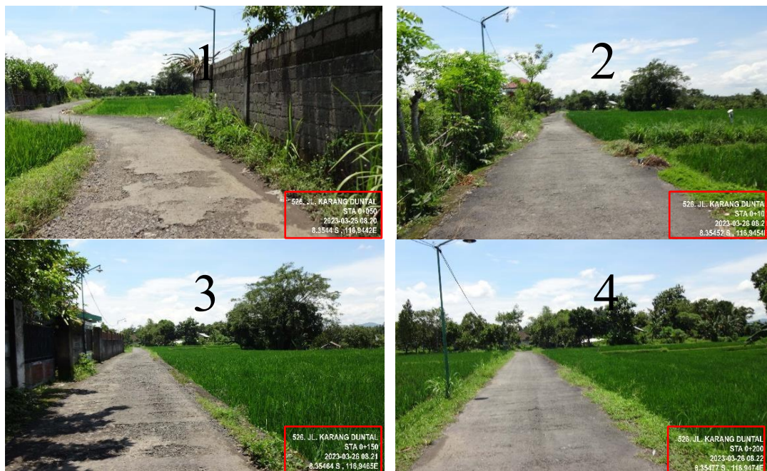
Fig. 4. Pictures of Road Surface Conditions on Jalan Karang Duntal.
