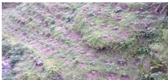
Fig.8. Photos of surface erosion appearance, (Source: Suwarno, 2014)
