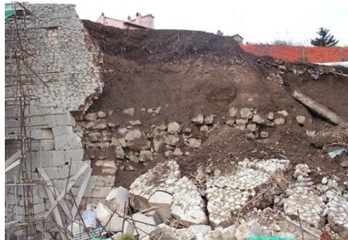
Fig. 12 Collapse in January 2006
