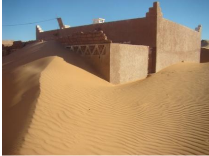
Fig. 5 One of silted habitations in Zaouïa, In-Salah (photo crstra, 2013)
